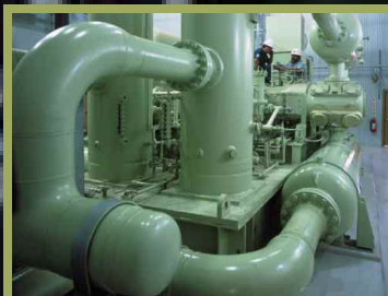
The new Sylmar compressor station is part of an aggressive expansion program at SoCalGas that increased capacity and supply of natural gas into Southern California by 11 percent in 2002.
