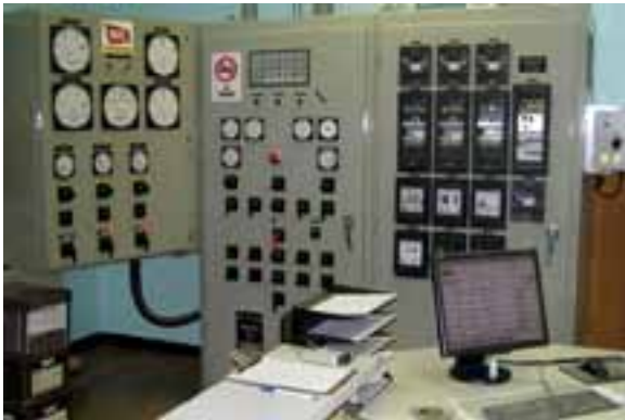
Control room at the BESS installation in Metlakatla, Alaska
