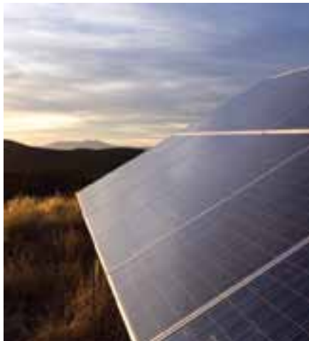
The Absolyte® GP battery serves as the energy storage system at this photovoltaic installation on Carol Spring Mountain in Globe, Arizona
