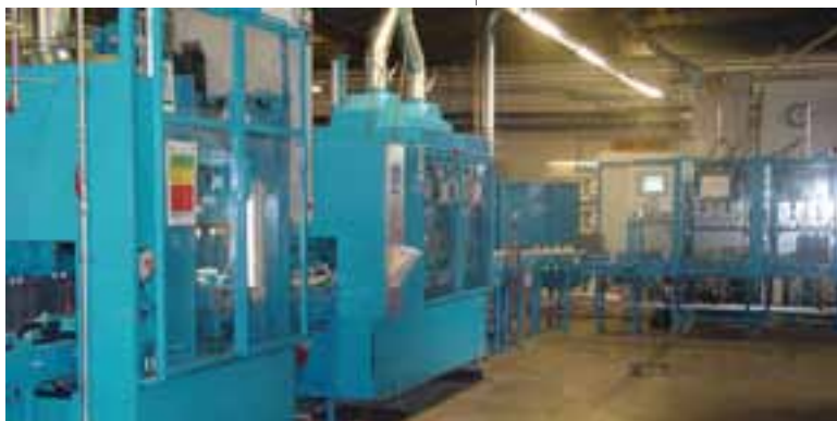
Upgraded and improved assembly line installation at the Exide Network Power manufacturing facility in Bűdingen, Germany
