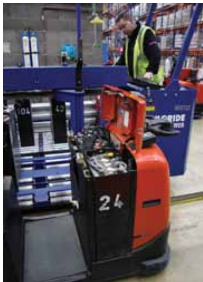
Battery changeout at Sainsbury's distribution center in Swan Valley, Northampton, UK
