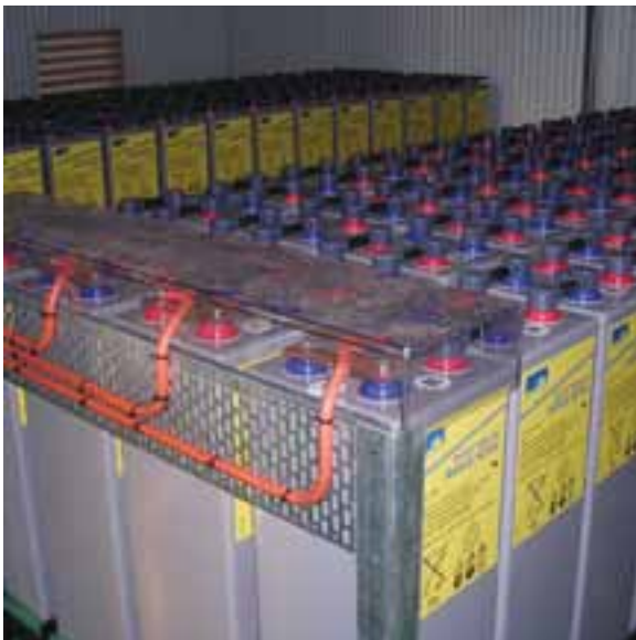
Sonnenschein® A600S battery installation providing sustainable energy at remote Bushlight communities across Australia
